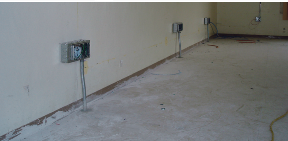
Computer Lab Junction Boxes
