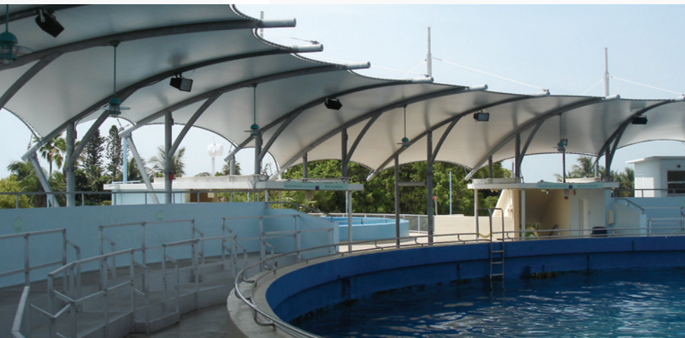
Canopy Structure with Wire Conduit
